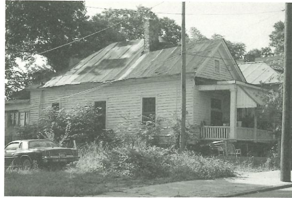
Signs of neglect are evident in many neighborhoods.
